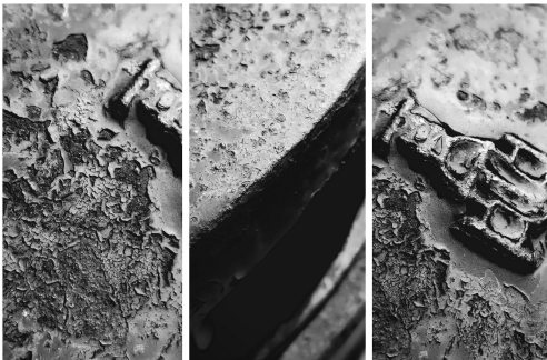
Fig.1 Fire Hydrant with rust
